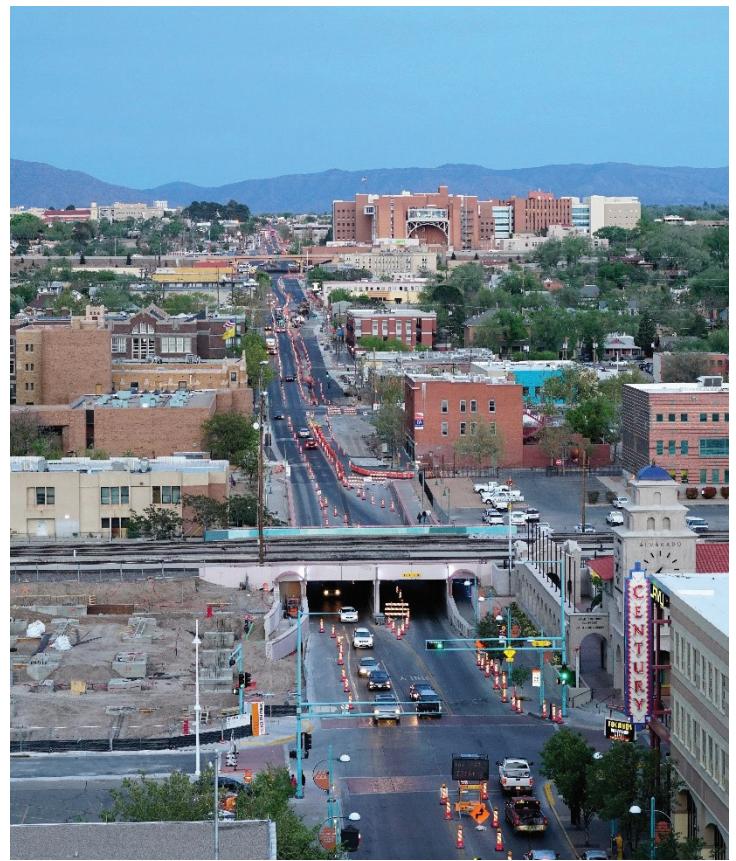
Albuquerque Rapid Transit construction on Central Avenue. Credit: samat k jain via Flickr, CC BY-SA 2.0.
